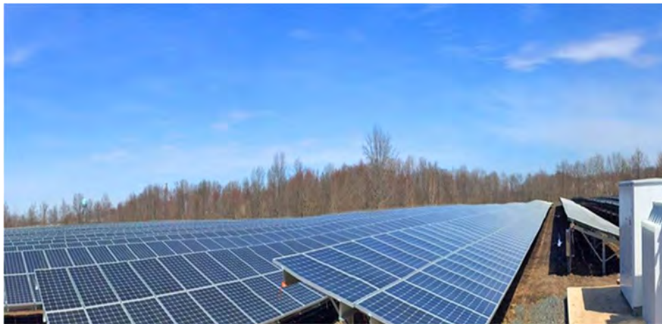
The 15MW Chambersburg Solar Center, on W. Commerce Street, in Hamilton Township, was completed in 2022 in partnership with Safari Energy, and sold to Aspen Power in 2023, provides affordable and reliable clean energy
